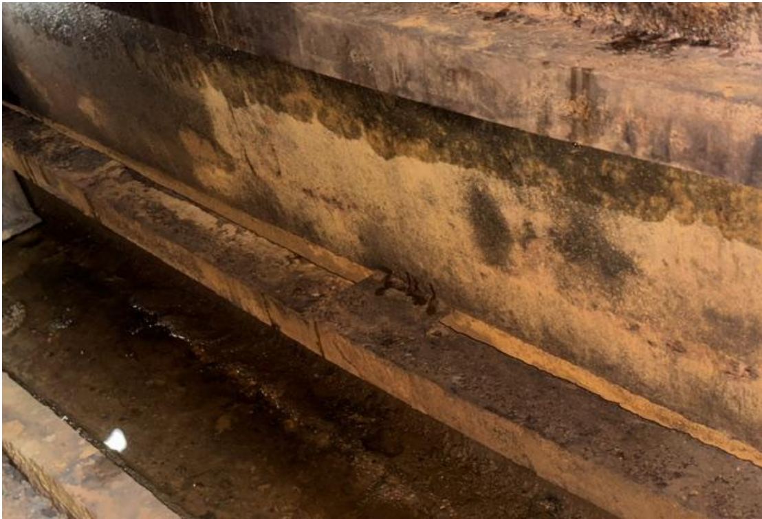
SIDE LONGITUDIANL NO. 4 WELDED TO BRACKETS NOT PLATING
