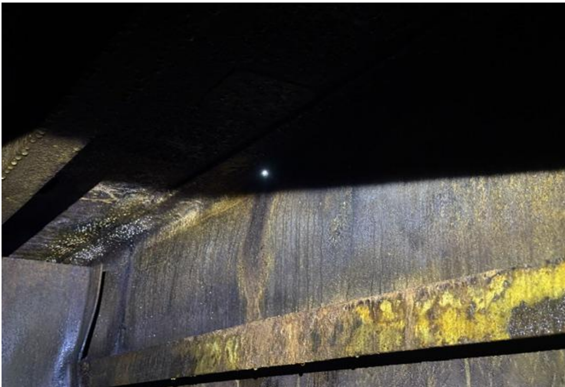
STARBOARD NO. 2 COMPARTMENT WITH PIN HOLE
