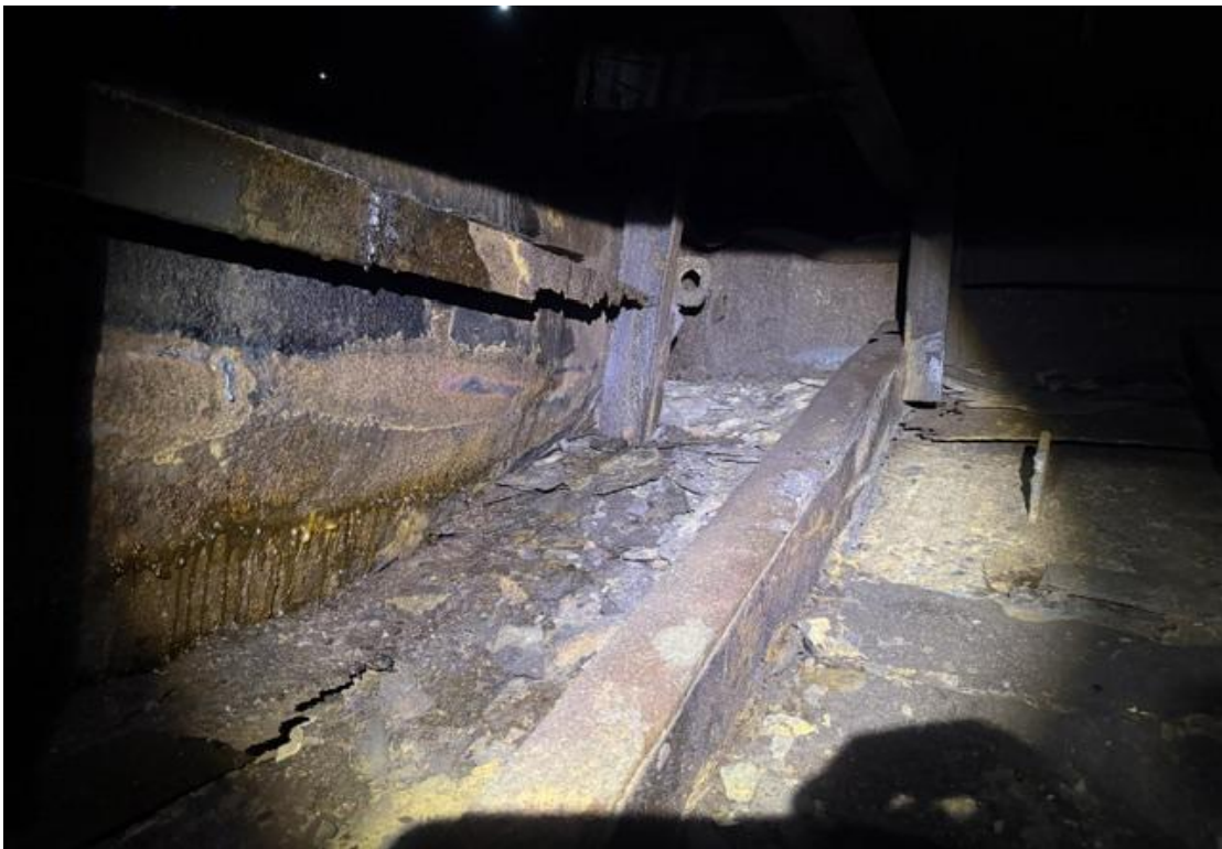
STERN RAKE COMPARTMENT SIDE LONGITUDINAL WITH WASTAGE
