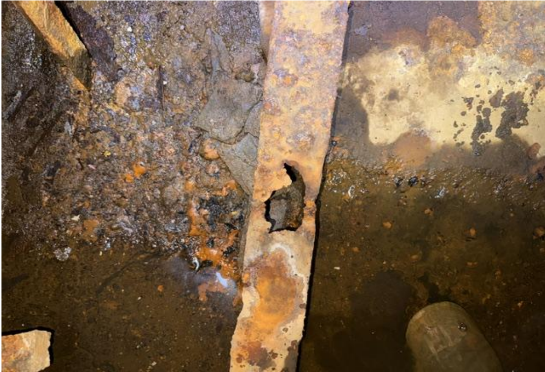
STERN RAKE COMPARTMENT BOTTOM LONGITUDINAL WITH WASTAGE
