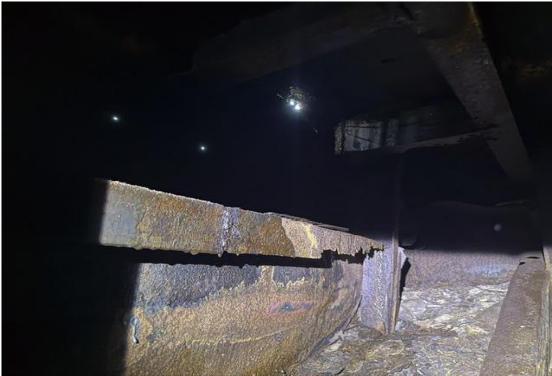
STERN RAKE COMPARTMENT STARBOARD SIDE PLATING CONTAINS HOLES
