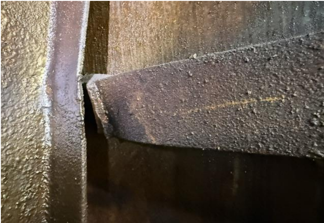
STARBOARD NO. 2 CONPARTMENT SIDE LONGITUDINAL WITH BROKEN WELD AT CHORD
