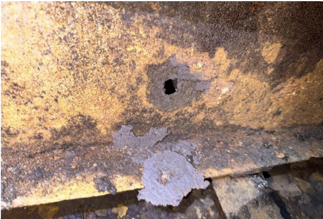
STERN RAKE COMPARTMENT BOTTOM CHORD WITH WASTAGE
